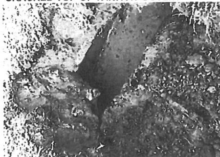
CRACKED TOP OF TANK AT OUTLET
