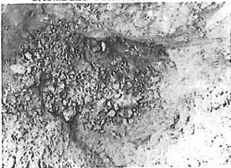
CRUMBLED CONCRETE DBOX
