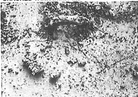
CRACKED TANK INLET LID
