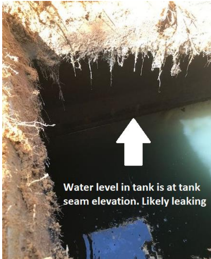
Figure 2. Inlet side of tank (leaking)
