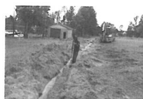
lozynski Repair 10-25-18 Gar
