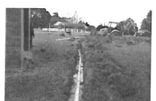
lozynski Repair 10-25-18 Gar
