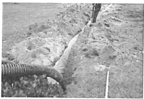
lozynski Repair 10-25-18 Gar
