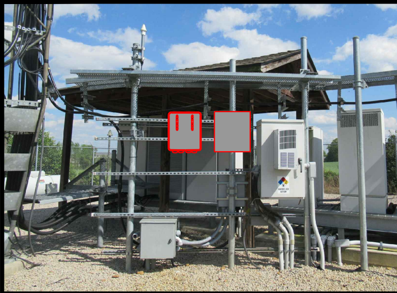
EXISTING USCC RRU RACK (FRONT)
