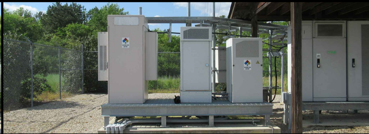
EXTERIOR USCC EQUIPMENT PAD #2
