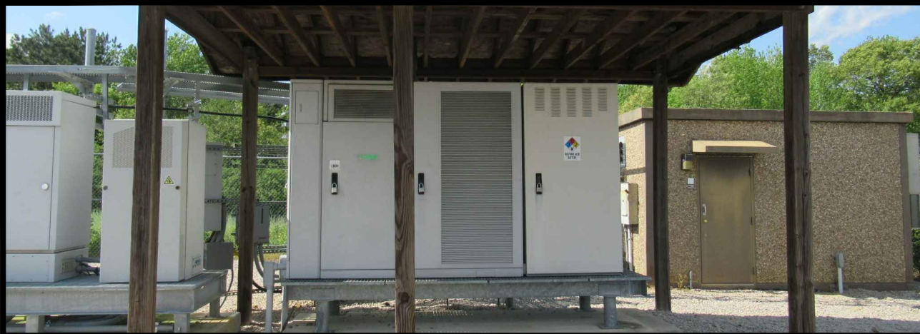
EXTERIOR USCC EQUIPMENT PAD #1
