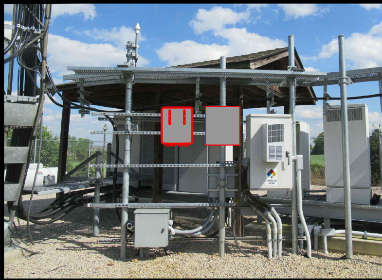
EXISTING USCC RRU RACK (FRONT)
