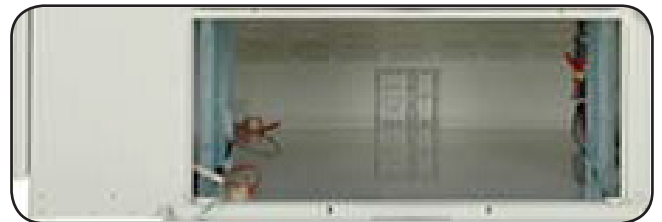
Battery Compartment (rear)
