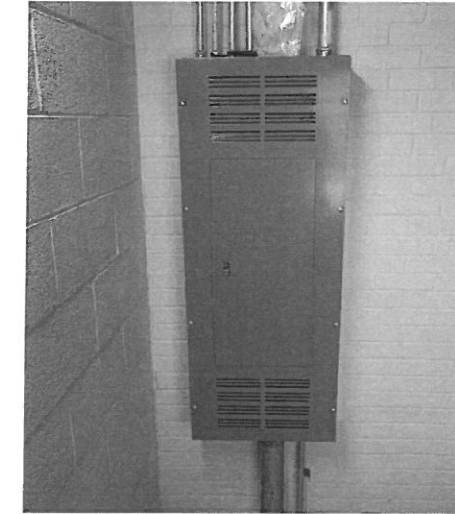
PHOTO #1 - EXISTING ELECTRICAL PANEL IN THIRD FLOOR STORAGE ROOM.
