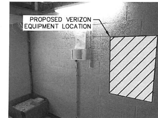
PHOTO #2 - PROPOSED LOCATION OF NEW VERIZON EQUIPMENT IN THIRD FLOOR STORAGE ROOM.
