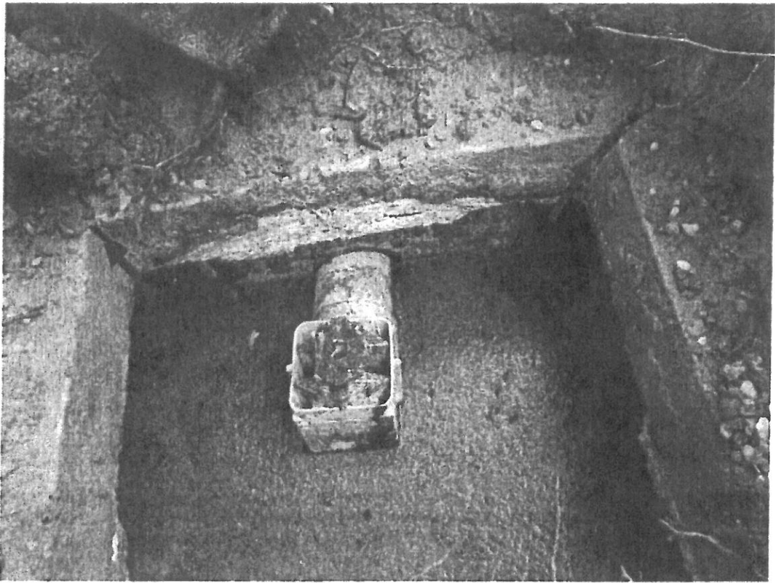
Cracks in Septic Tank
