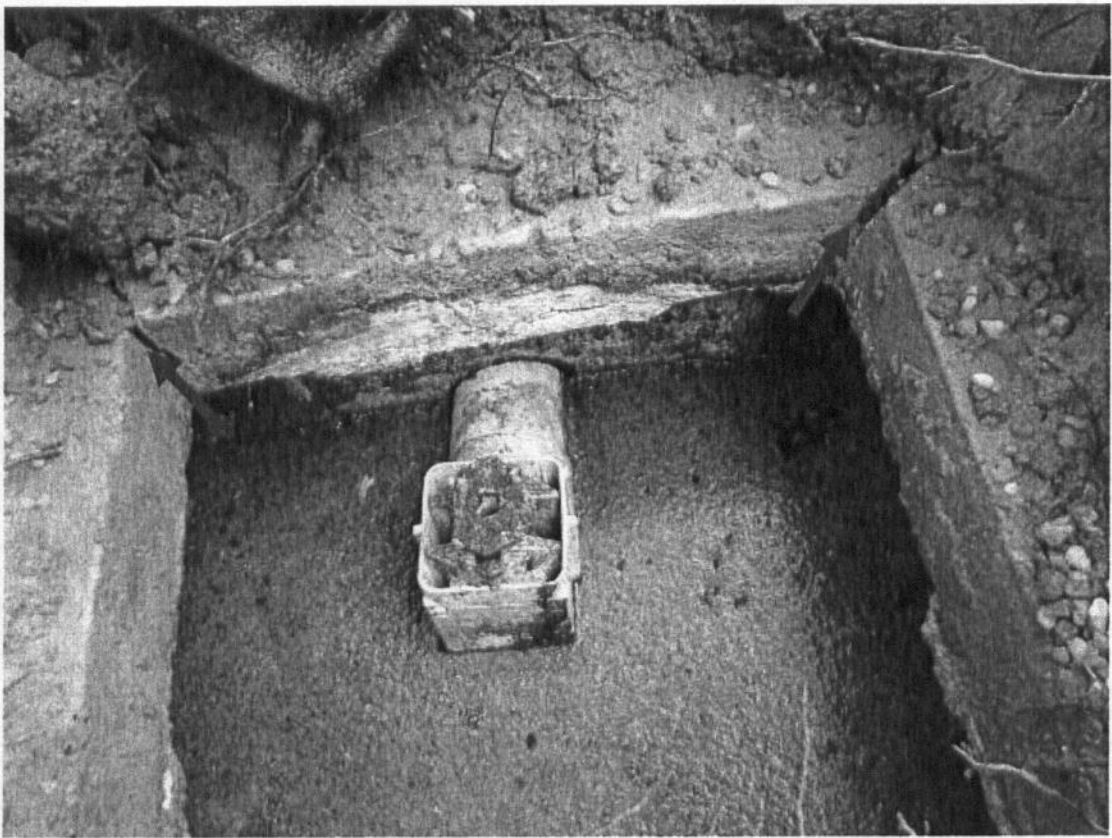
Cracks in Septic Tank
