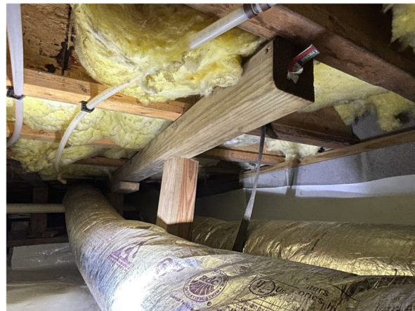
Picture 4 – Improperly constructed support
