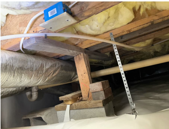
Picture 3 – Improperly constructed support
