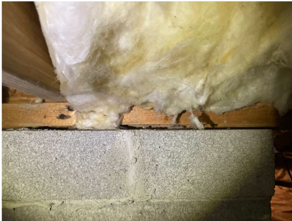
Picture 3 – Out-of-contact masonry pier
