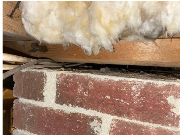
Picture 4 – Out-of-contact masonry pier
