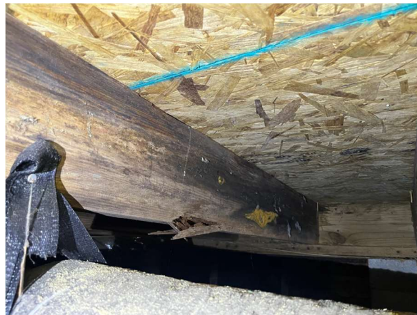
Picture 3 – Example of a cracked joist
