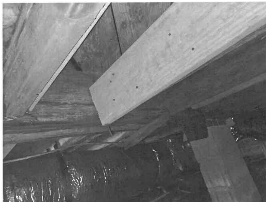
Picture 4 – Improperly reinforced joist
