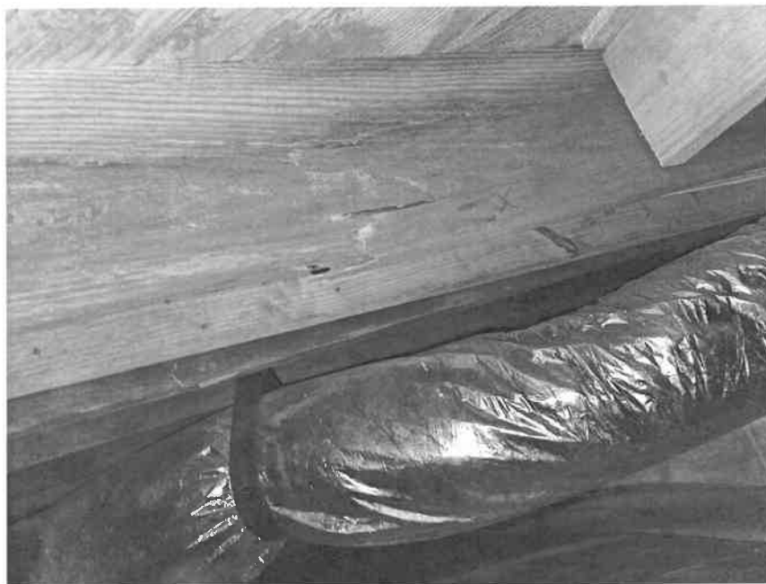
Picture 3 – Deteriorated joist
