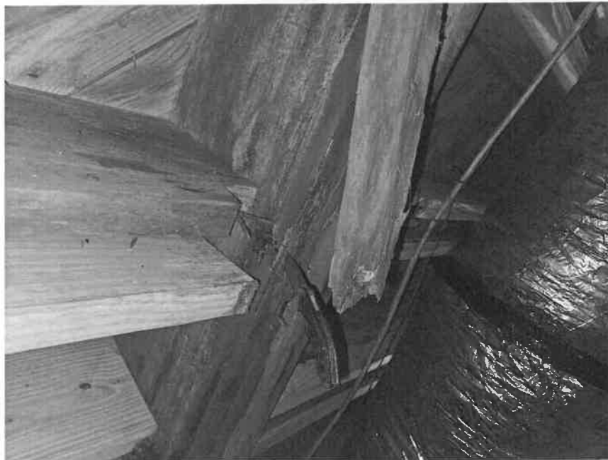
Picture 2 – Deteriorated girder and ledger strip
