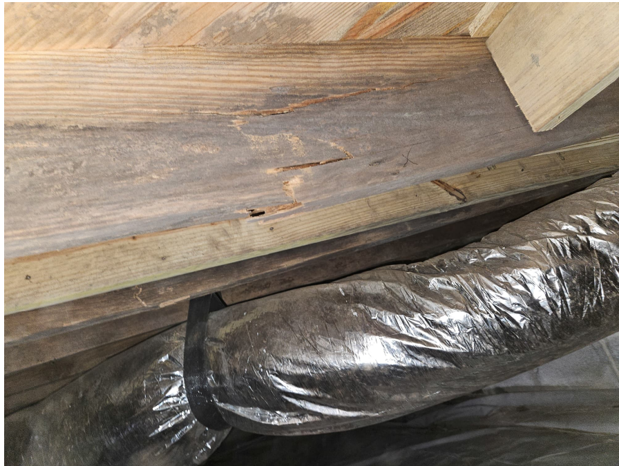
Picture 3 – Deteriorated joist
