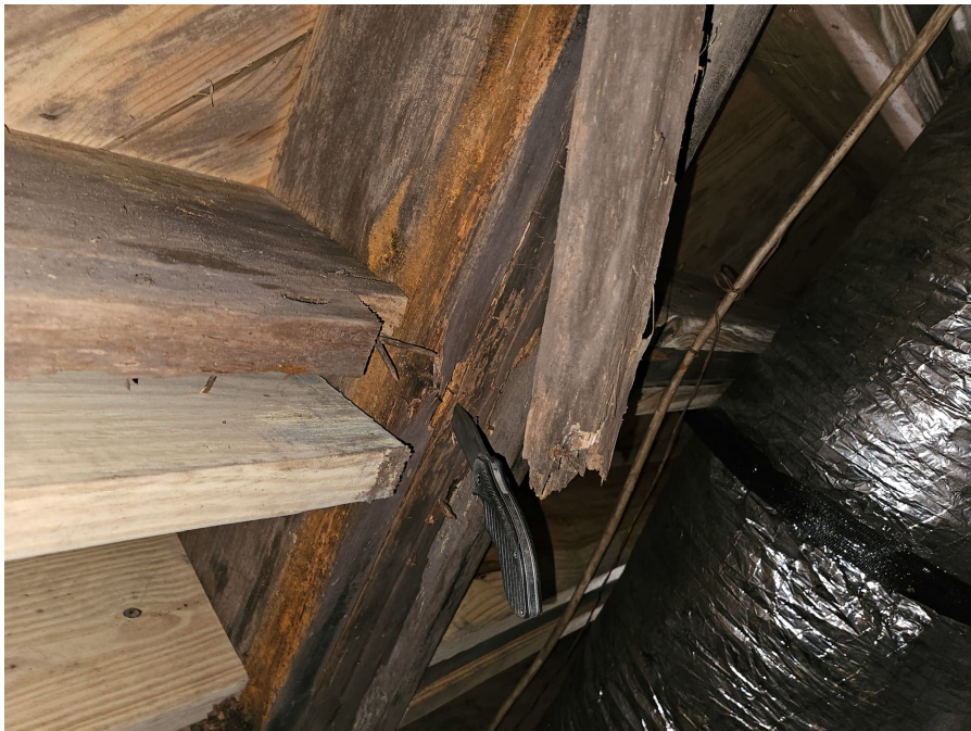
Picture 2 – Deteriorated girder and ledger strip
