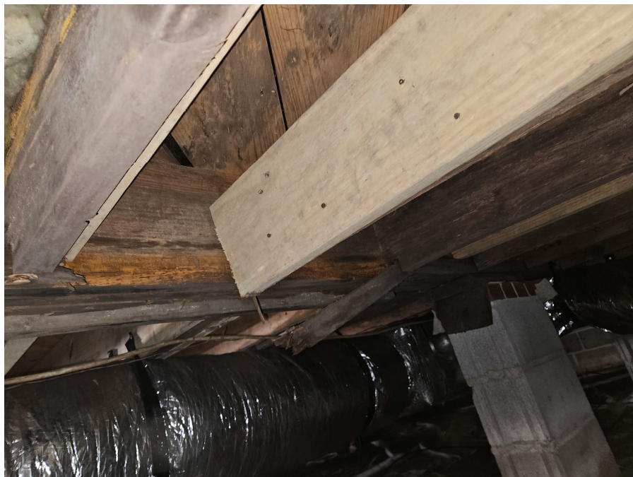
Picture 4 – Improperly reinforced joist
