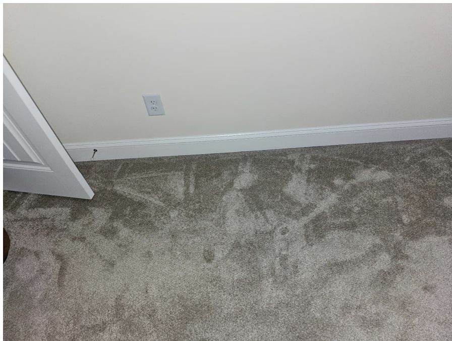
Picture 2 – Area of creaking floors in the primary bedroom
