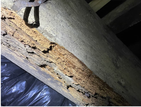
Picture 3 – Deteriorated girder
