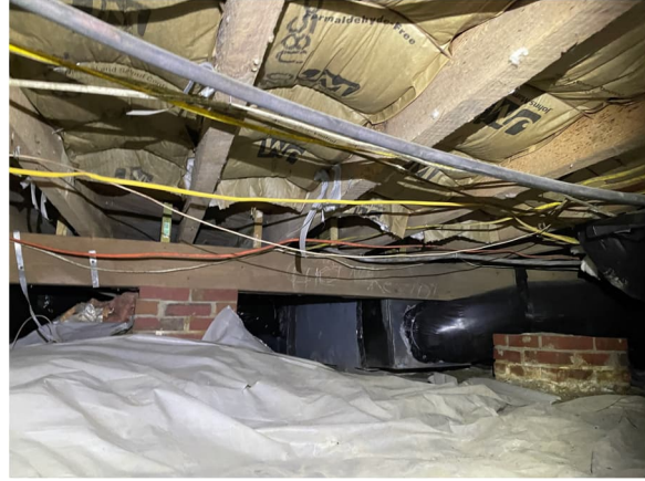
Picture 4 – Deteriorated joists
