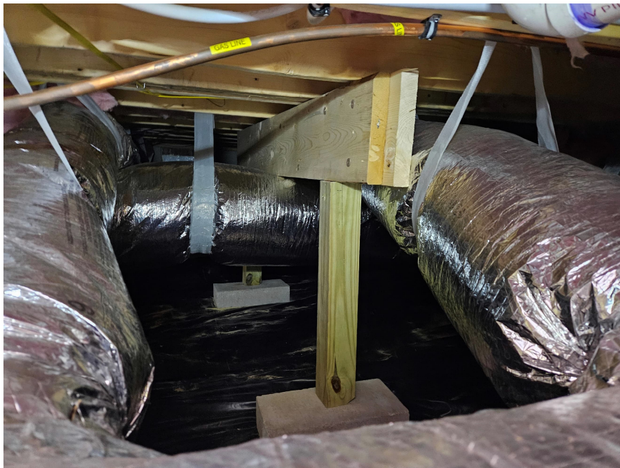
Picture 2 – Example of haphazard support
