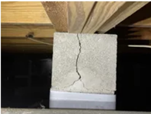
Picture 5 – Cracked CMU Block Supporting Girder
