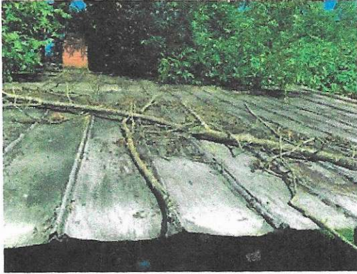
(14A) – Roof Coat Chrysotile 3%
