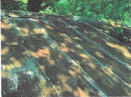
(16A) – Roof Coat Chrysotile 3%
