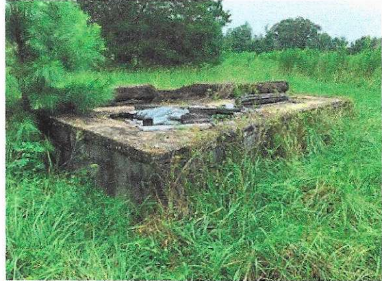
Septic/Water Storage Tank
