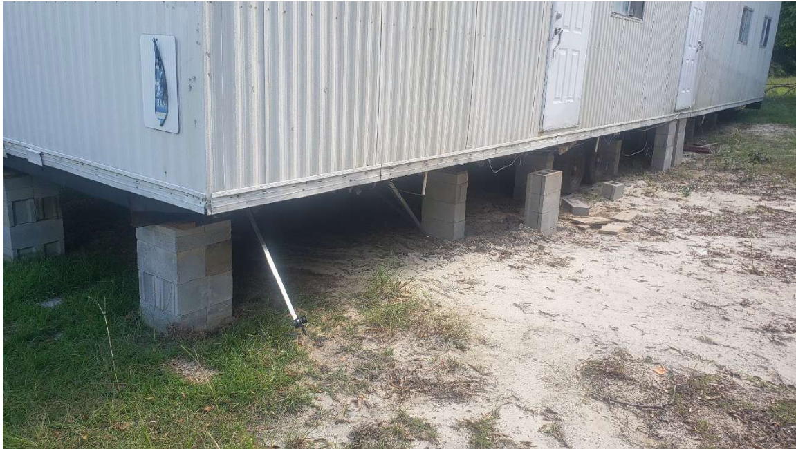
Example of straps installed per previous report
