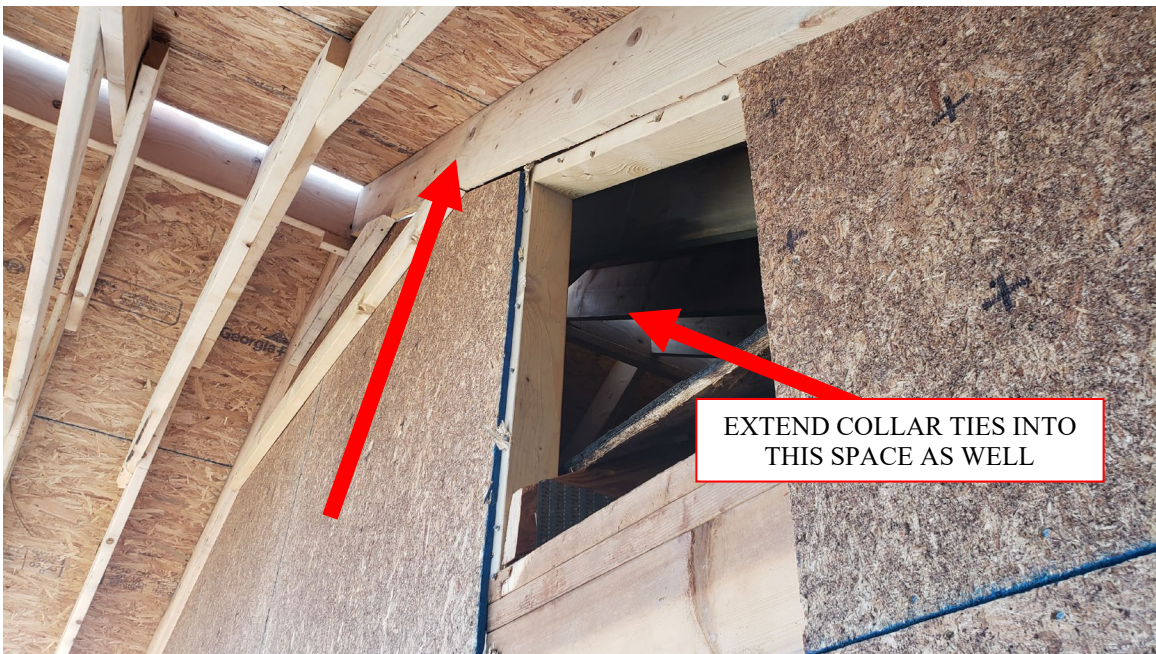
Example of collar ties to be installed per item 1.a of report
