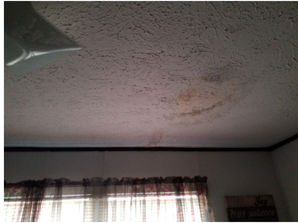
002D, 002 - Textured Ceiling, Bedroom 3, Main Floor
