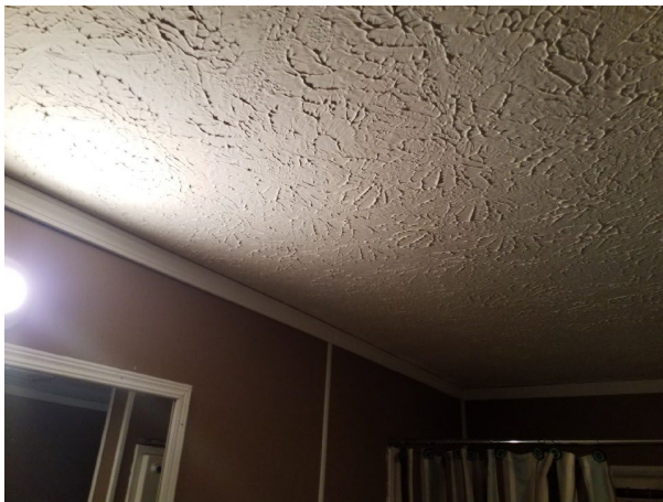
002E, 002 - Textured Ceiling, Bathroom 2, Main Floor
