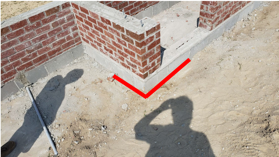
Item 1) Approximate locations of inadequate projection (red)
