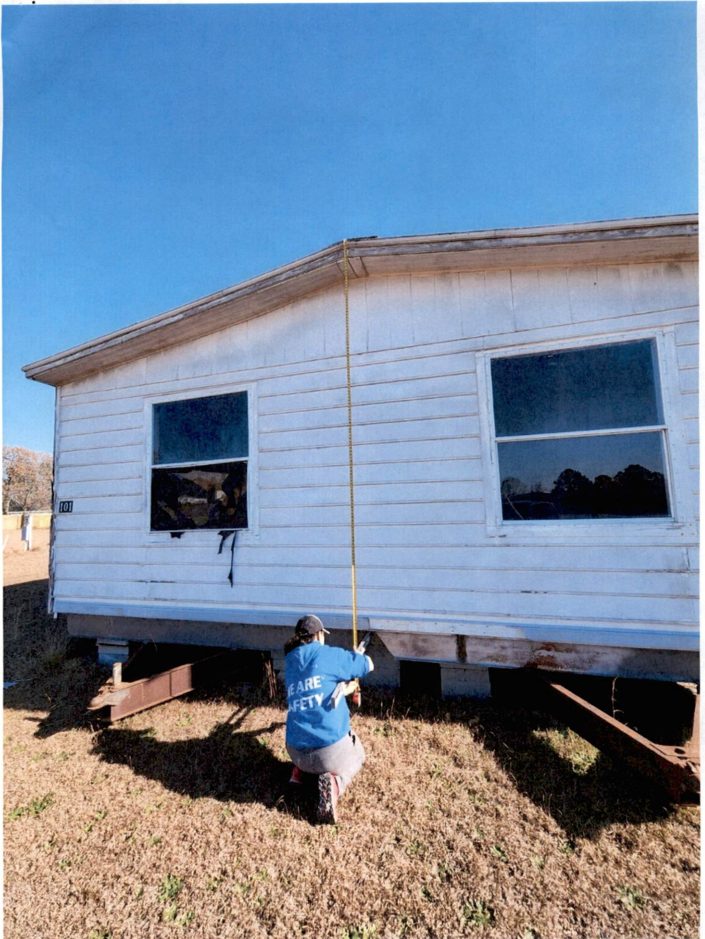
We plan on installing new shingles to extend to the required code of 12" pitch overhang as well as installing a front porch of 6'x8'.
