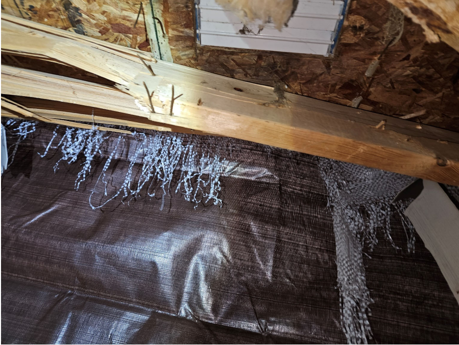
Picture 4 – Damaged framing
