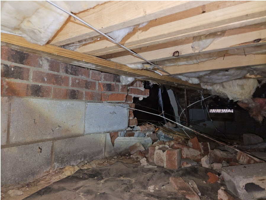
Picture 3 – Damaged foundation
