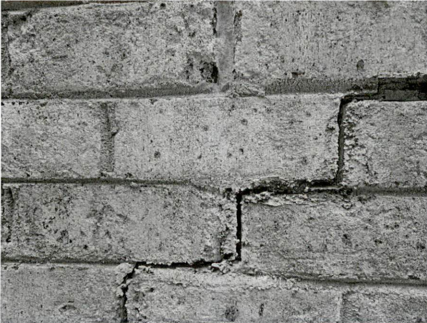
Picture 3 – Example of perimeter crack
