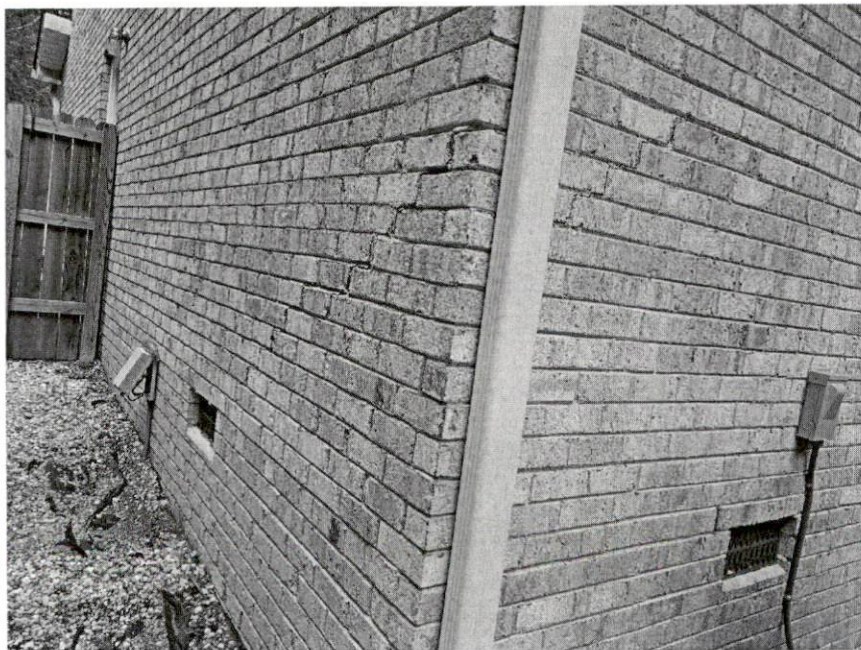
Picture 2 – Example of perimeter crack
