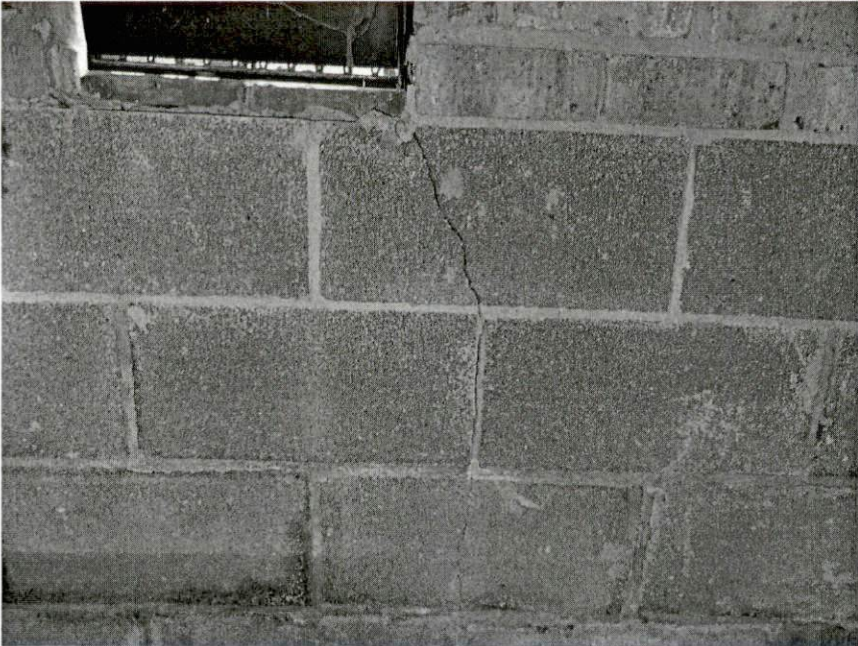
Picture 4 – Example of perimeter crack
