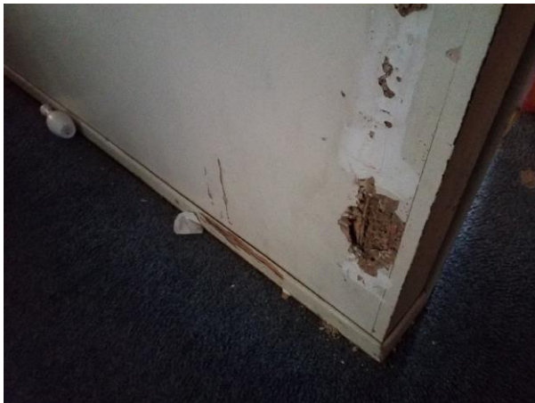
004A, 004 - Gypsum Wallboard System (Wallboard, Joint Tape, and Joint Compound), Hallway, Main Floor
