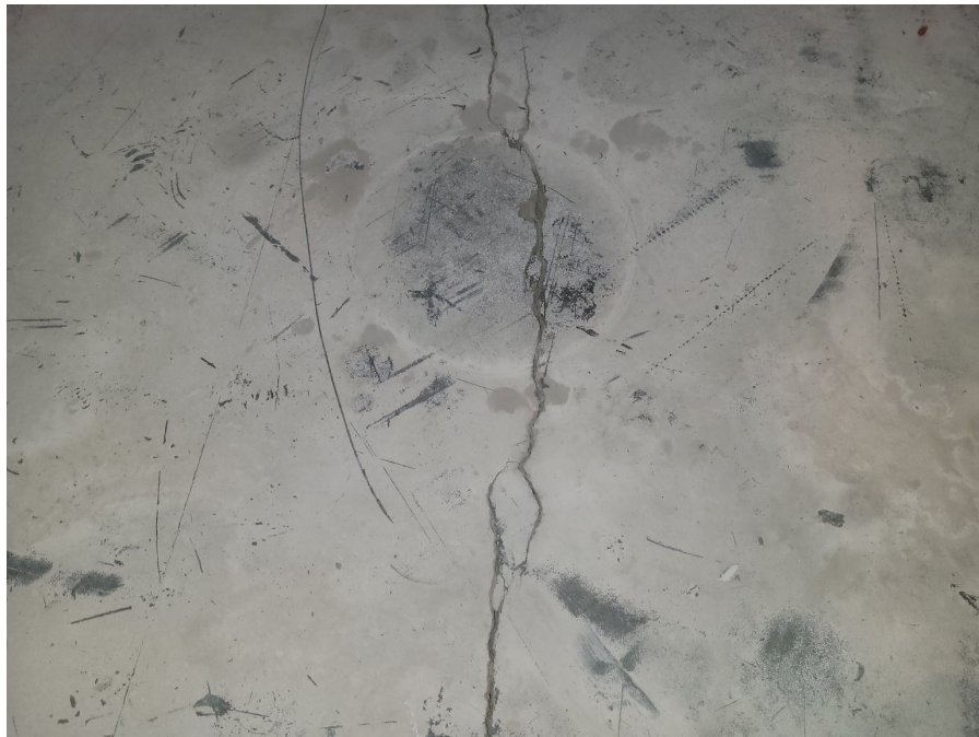
Picture 4 – Example of basement slab crack “feathering”
