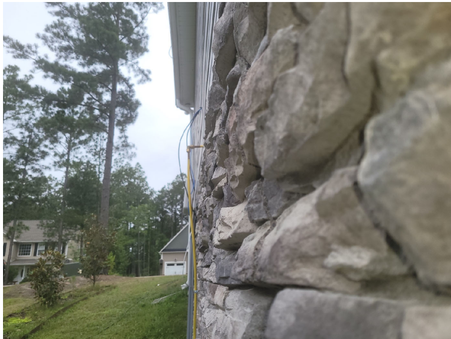
Picture 6 – Stone veneer offset across crack
