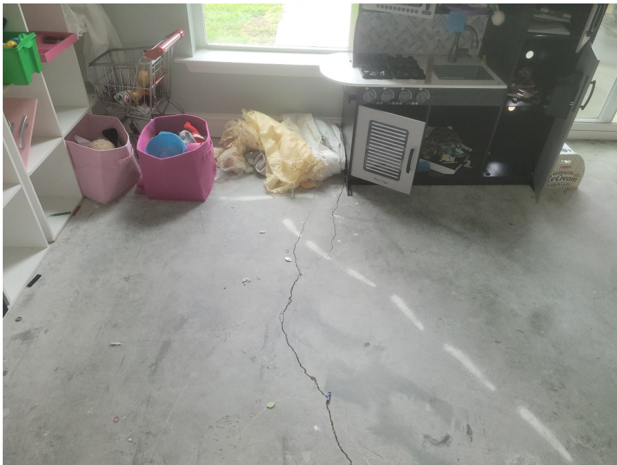
Picture 2 – Basement slab crack
