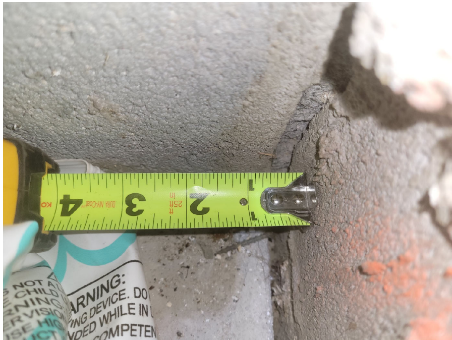
Picture 8 – Visibly shifted foundation wall at corner of garage
