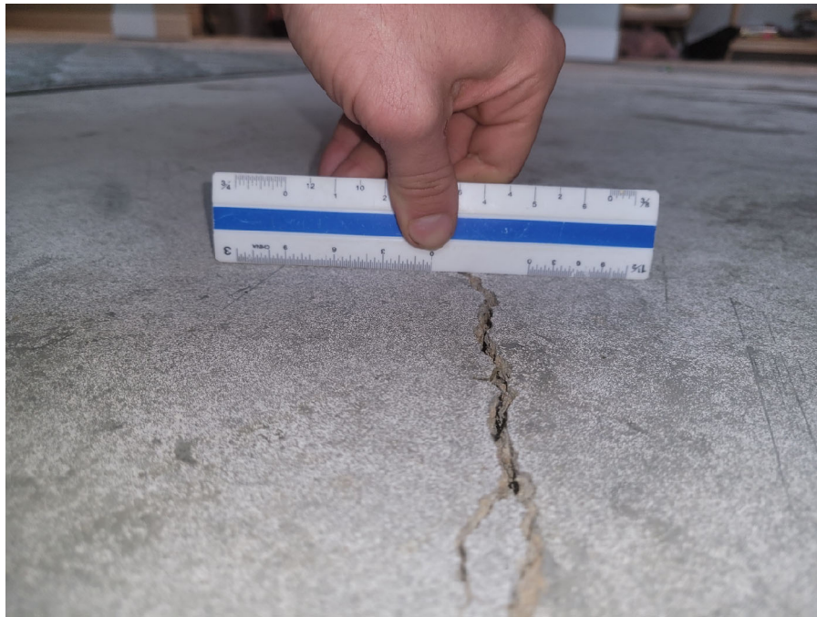
Picture 3 – Example of basement slab flush across crack
