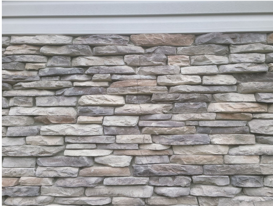
Picture 5 – Crack in stone veneer
