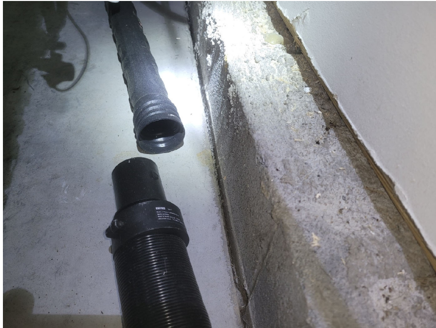
Picture 7 – Gap between garage slab and foundation wall
