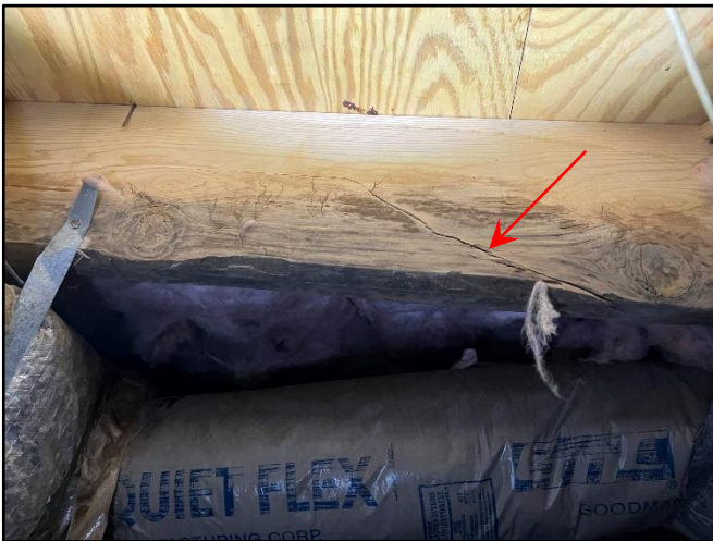
Photo 3 Deteriorated floor joist.
