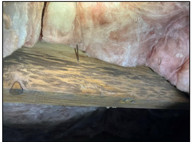
Photo 4 Deteriorated floor joist and biological growth.
