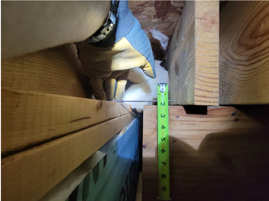
Picture 3 – Example of girder set low to the perimeter sill plate
