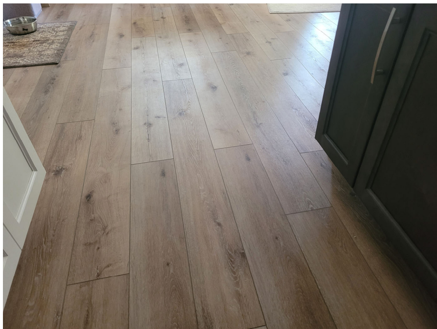
Picture 6 – Example of dip in floors at kitchen island
