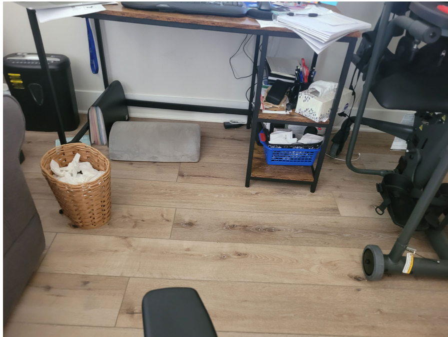
Picture 9 – Example of uneven floors in the office
