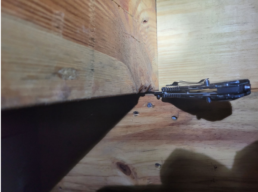
Picture 4 – Example of joist out of contact with the girder below
