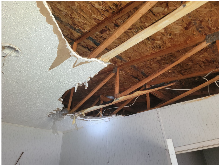
Picture 3 – Example of fire damaged roof truss
