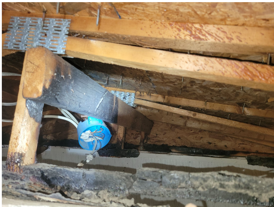
Picture 4 – Example of fire damaged roof truss
