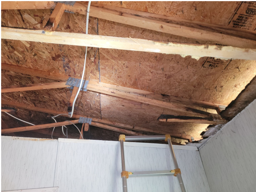
Picture 2 – Example of fire damaged roof truss
