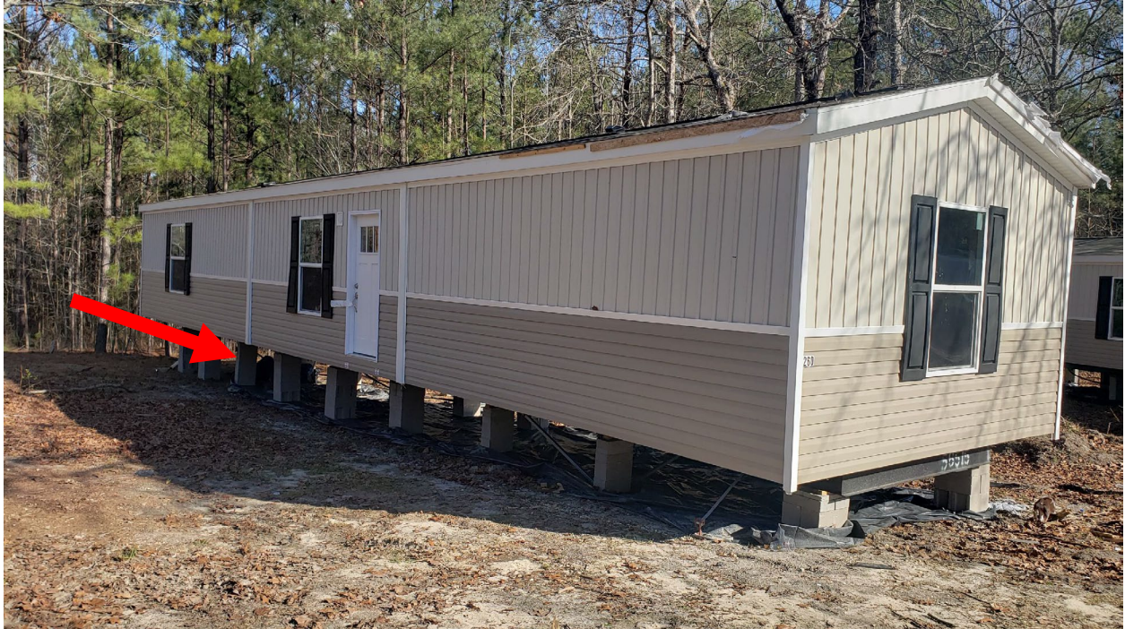
Site Inspected and 8" x 16" CMU pier to be replaced with new 16" x 16" CMU pier
