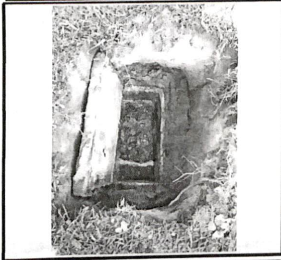
Distribution box showing sludge inside and needs to be cleaned out.
