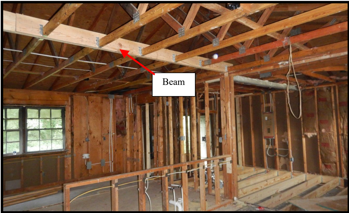
Photo #2 - This is a photo of the new beam that was added.
