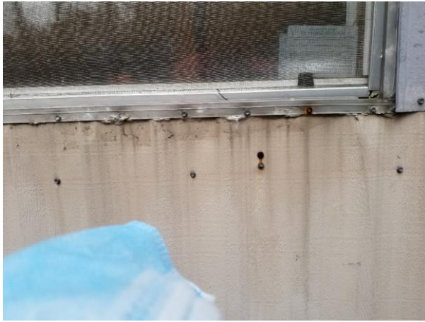
004A, 004 - Caulk, Window, Side A, Main floor
