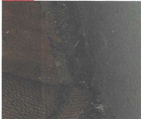
(11A,11B) – Sheetgood (Tan) Chrysotile 20% Mastic 2%
