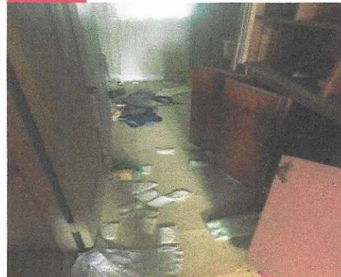
(10A,10B)-Sheetgood (Tan) Chrysotile 20% Mastic 2%
