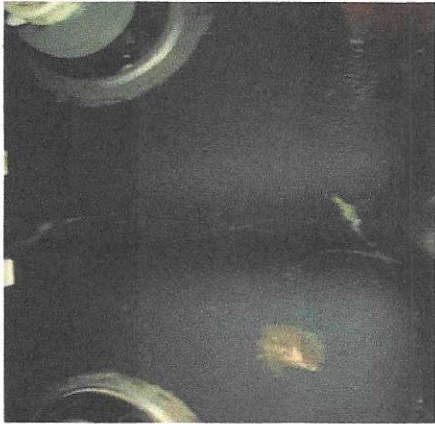
(13A) Sink Undercoat Chrysotile 5%
