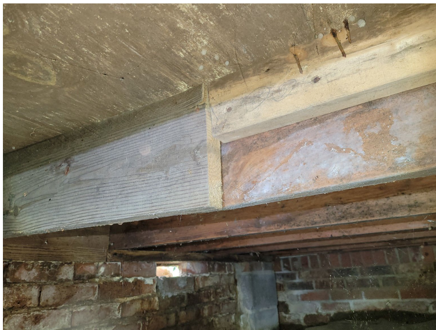
Picture 6 – Example of haphazardly reinforced floor joist
