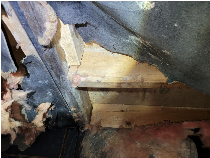
Picture 8 – Example of haphazardly replaced floor sheathing
