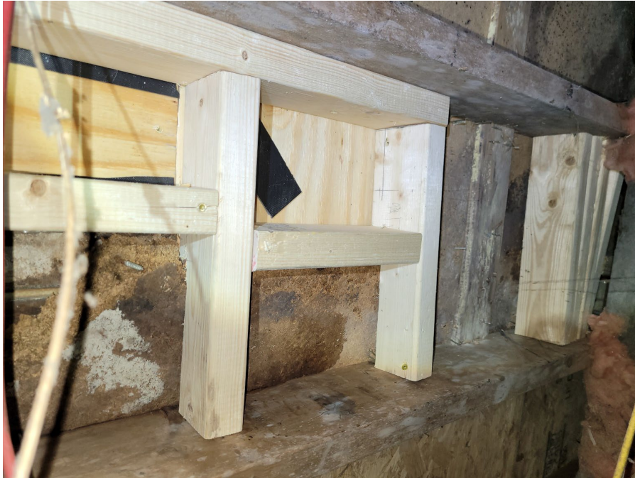
Picture 7 – Example of haphazardly replaced sheathing
