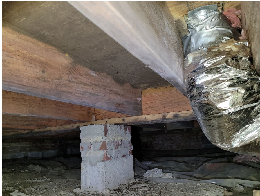
Picture 5 – Example of deteriorated floor joist
