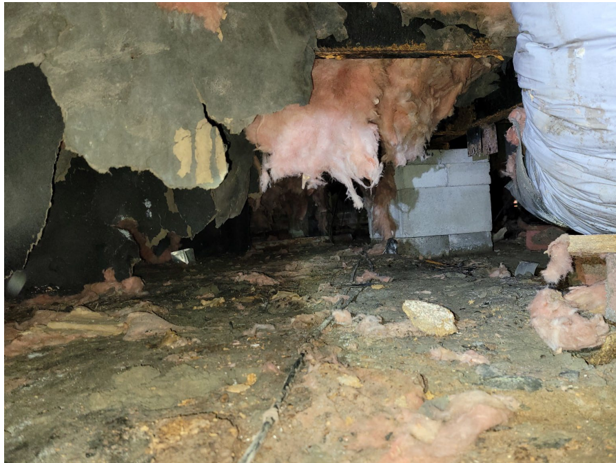
Picture 9 – Example of damp soils with poor vapor barrier coverage
