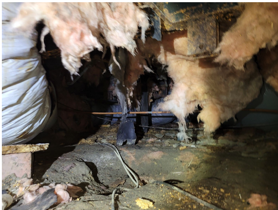
Picture 10 – Example of limited access due to clearance and ductwork
