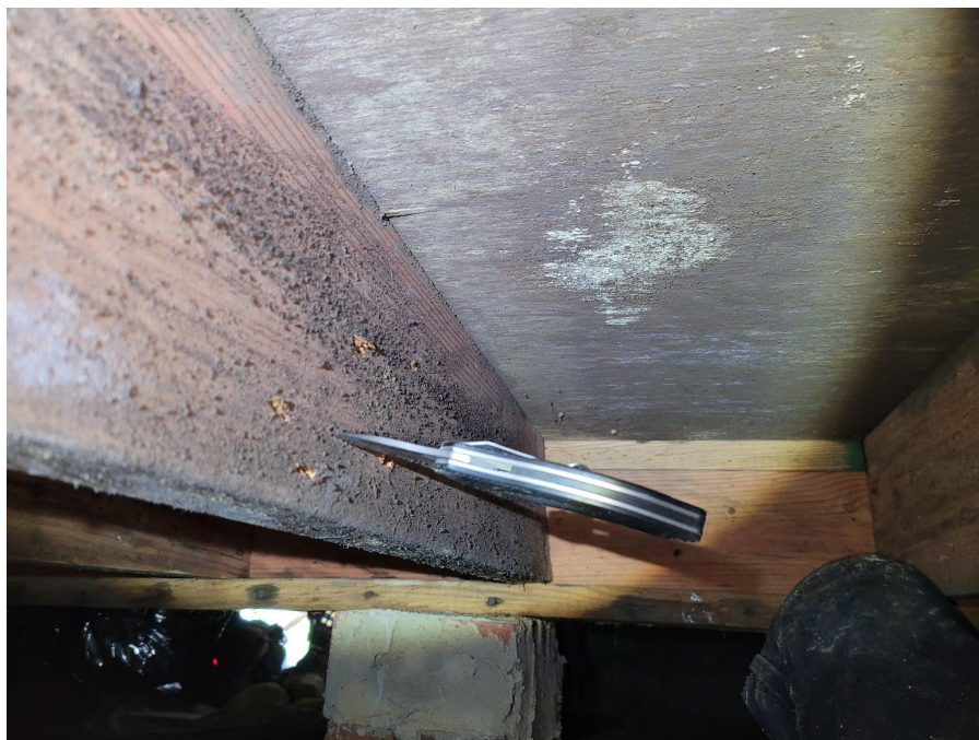
Picture 4 – Example of deteriorated floor joist
