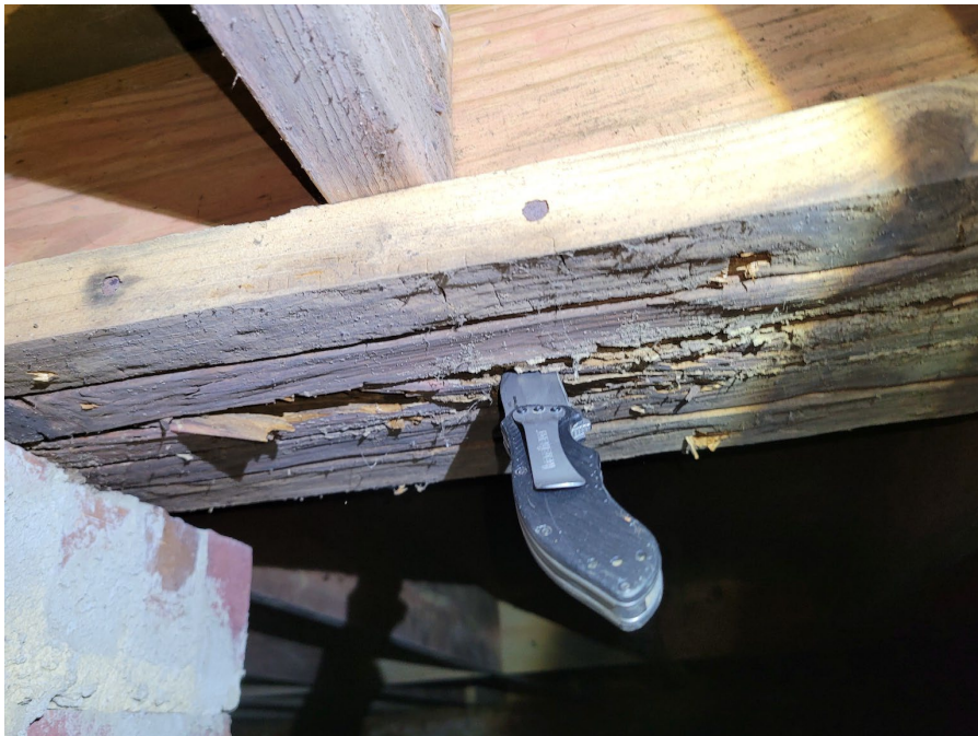
Picture 2 – Example of deteriorated girder
