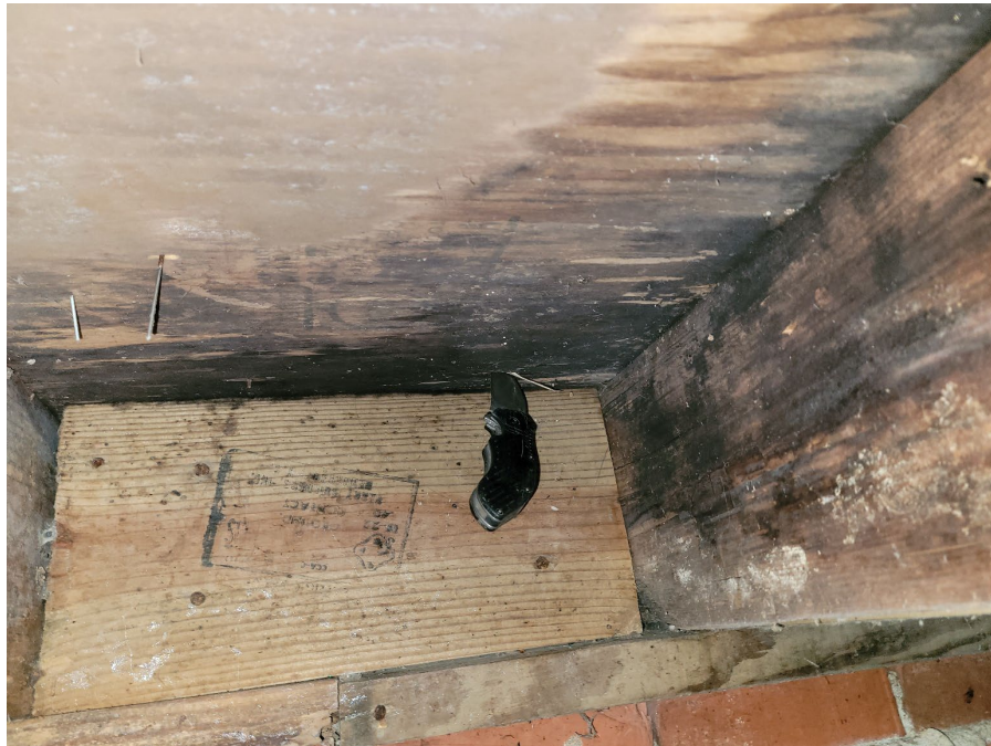
Picture 3 – Example of deteriorated sheathing
