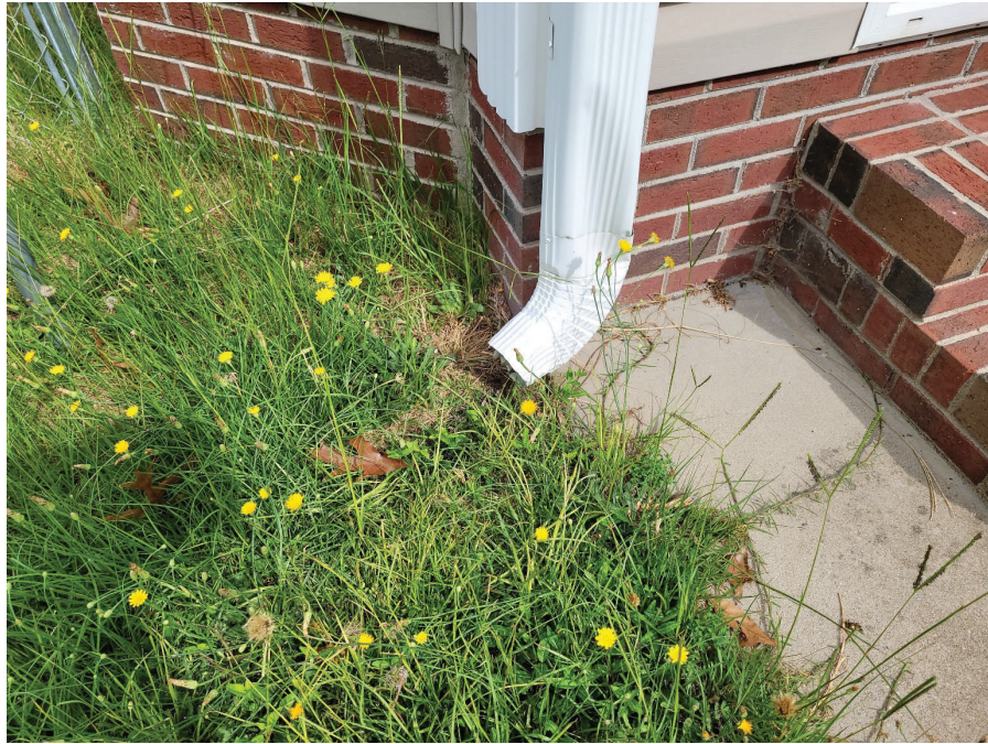
Picture 3 – Roof gutter downspouts installed for discharge at the foundation
