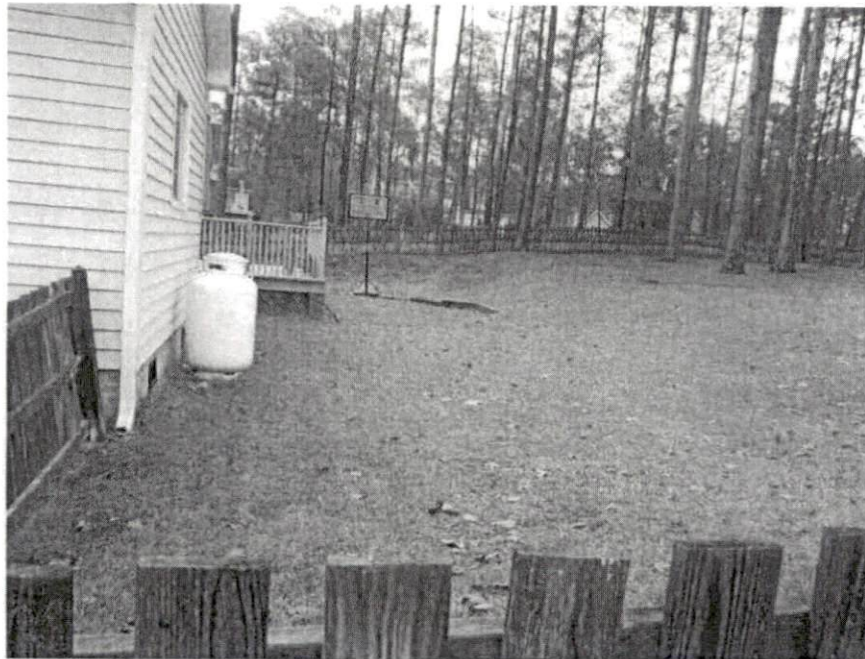
Picture 7 – Inadequately sloped exterior grade at back of home
