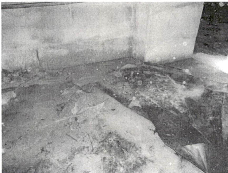
Picture 6 – Standing water at back foundation wall
