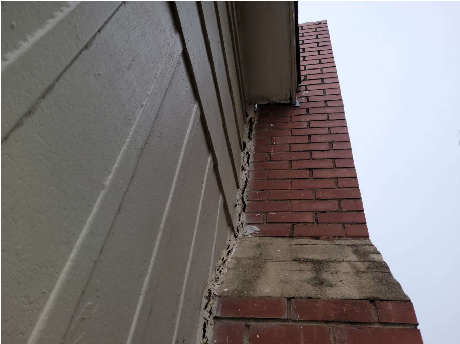
Picture 2 – Leaning chimney
