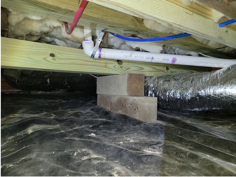
Picture 6 – Haphazardly constructed wooden support
