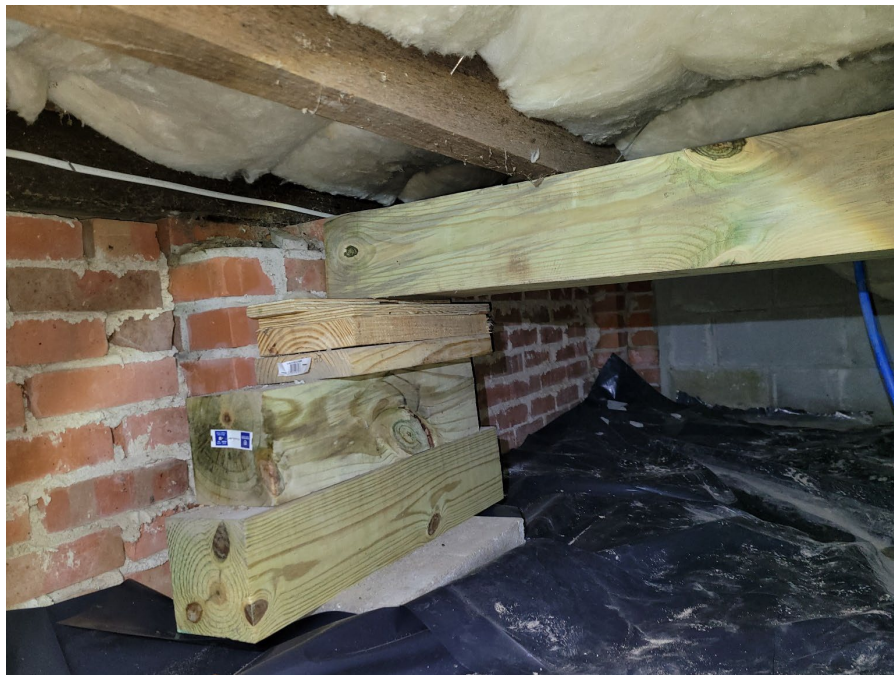
Picture 4 – Haphazardly constructed wooden support
