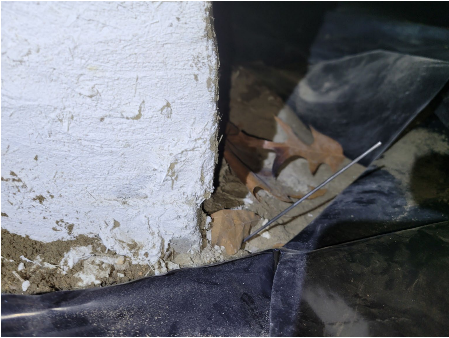
Picture 7 – New CMU pier with no footing
