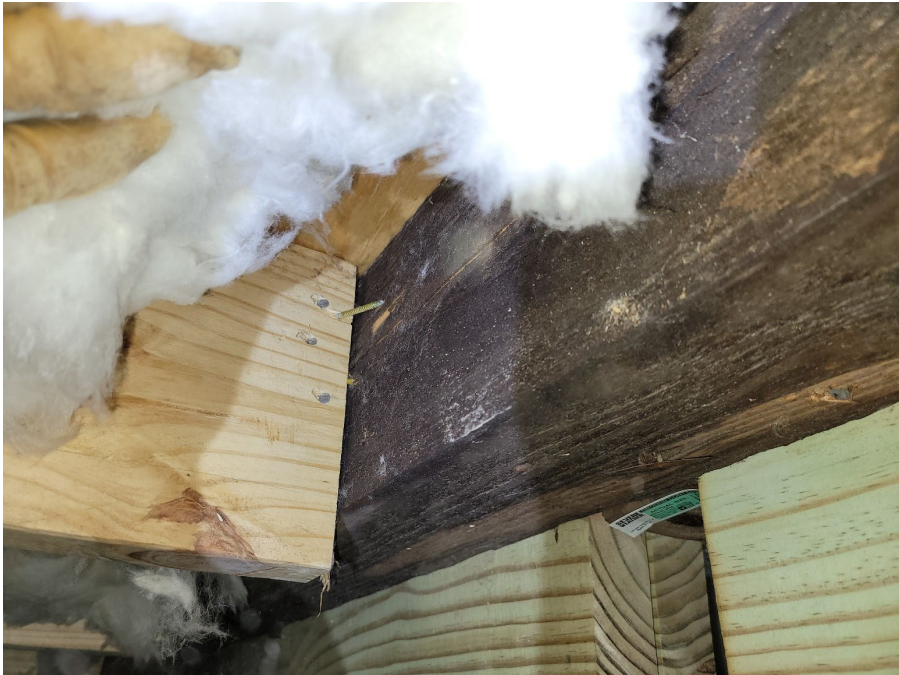
Picture 2 – New floor joist inadequately fastened to existing girder
