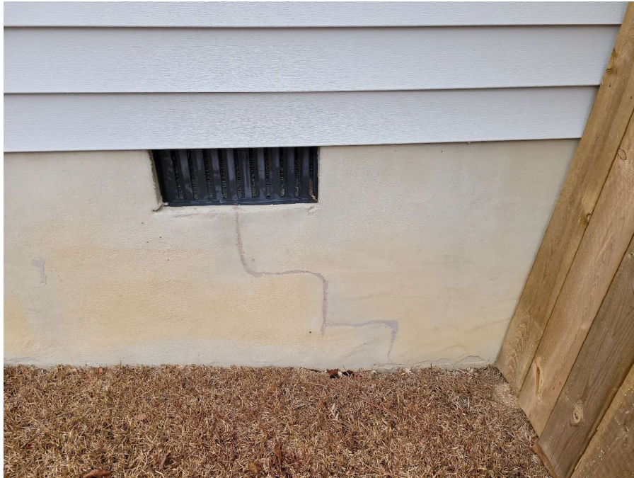
Picture 3 – Example of parging cracks
