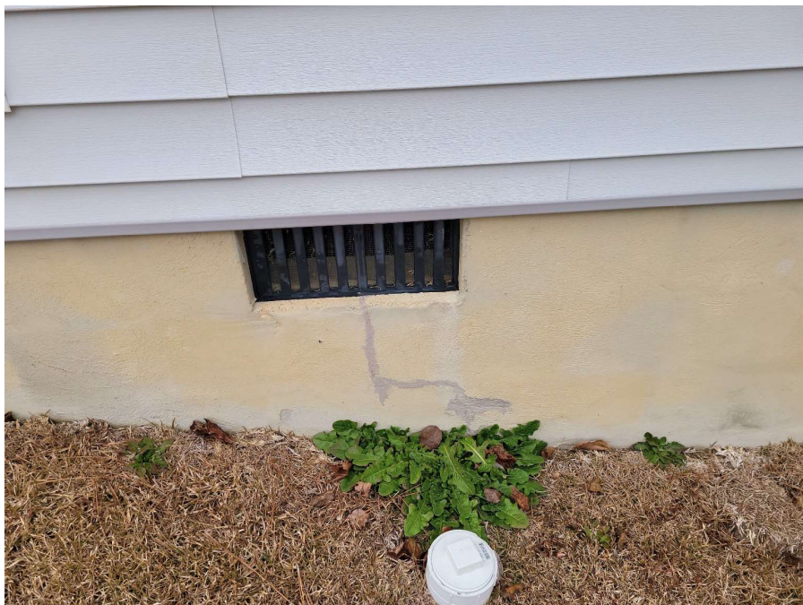
Picture 2 – Example of parging cracks
