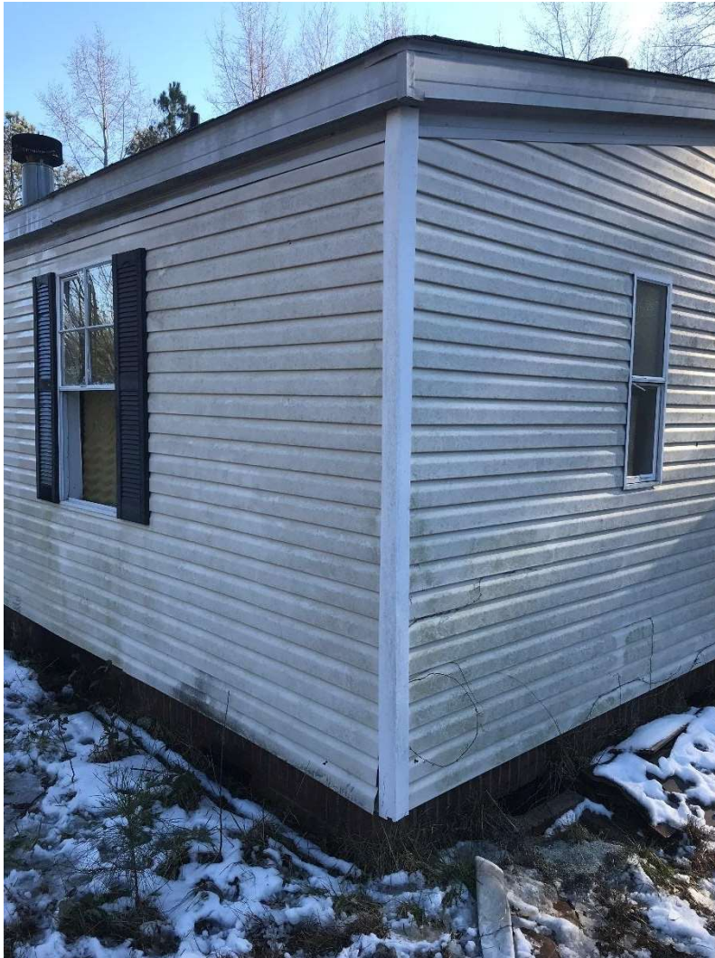
Figure 4. Lack of drainage management
