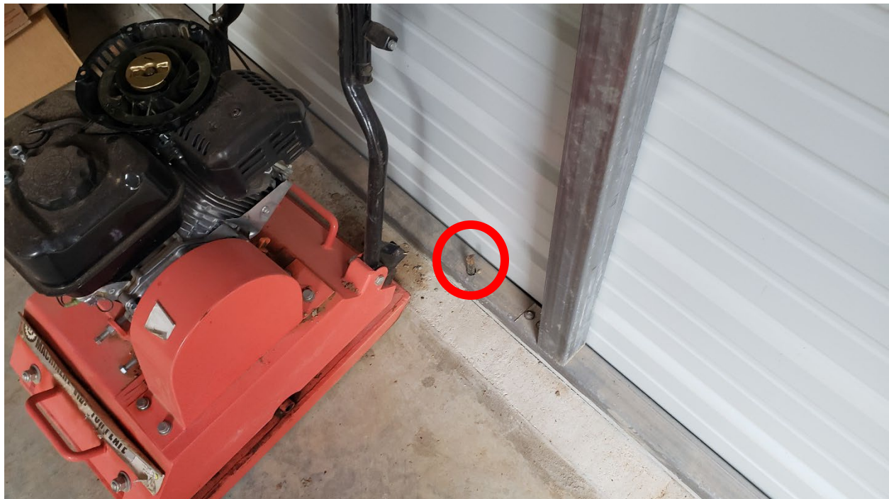
Example of inadequate anchoring configuration/rebar used
