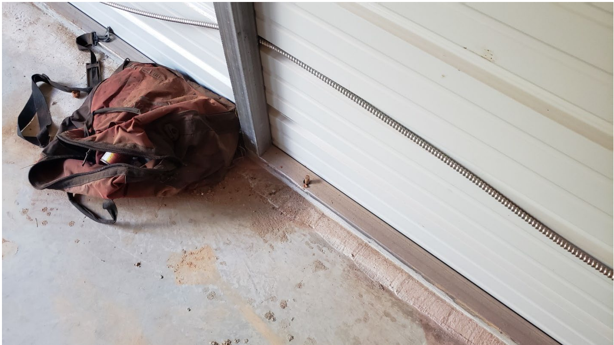
Additional examples of inadequate anchoring configuration/rebar used
