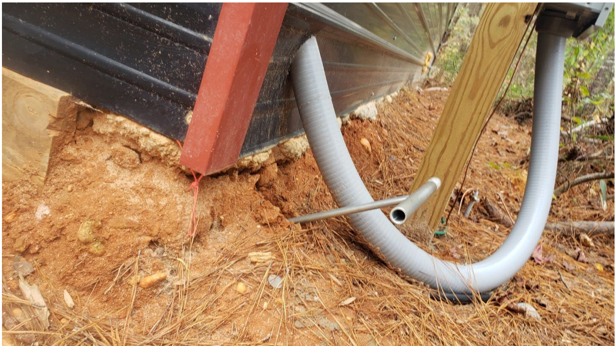
Example of missing/inadequate footings
