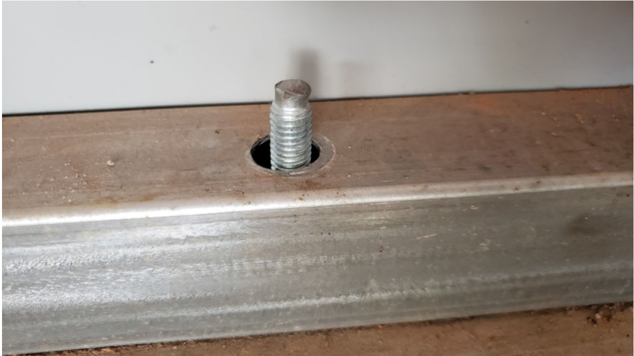
Examples of inadequate anchoring configuration/missing nuts and washers
