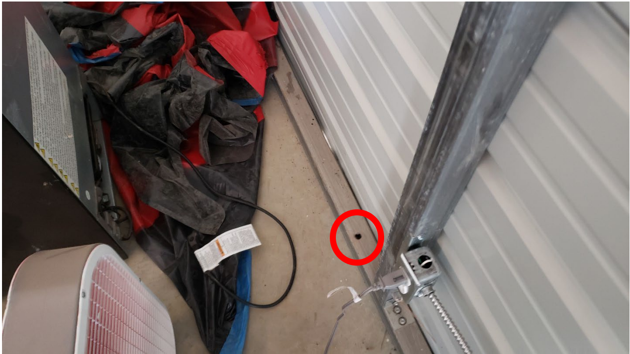
Examples of inadequate anchoring configuration/missing anchors
