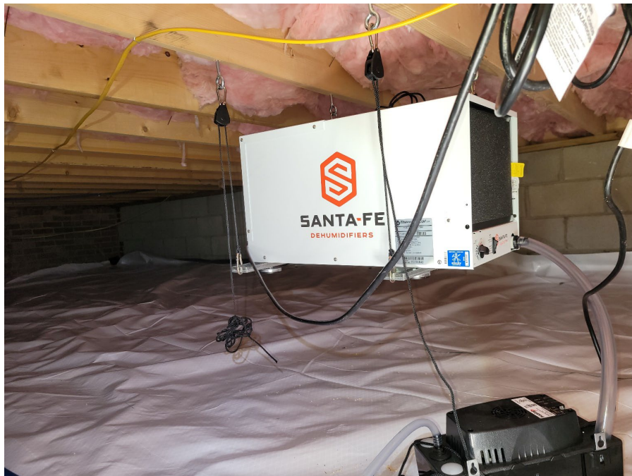
Picture 6 – Example of dehumidifier
