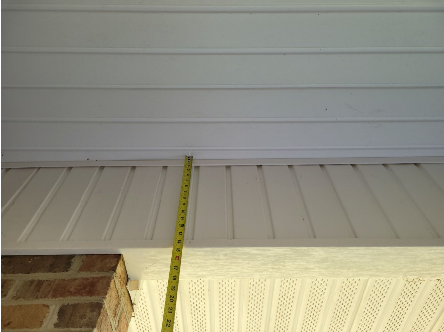
Picture 4 – Example of dropped beam supporting the front ends of the roof trusses
