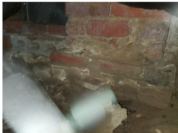
Picture 12 – Undermined pilaster at HVAC
