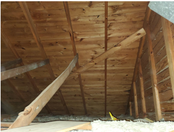
Picture 3 – Missing diagonal
