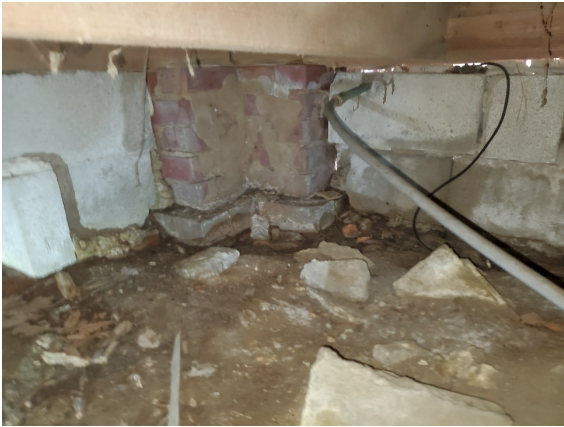
Picture 13 – Undermined pilaster
