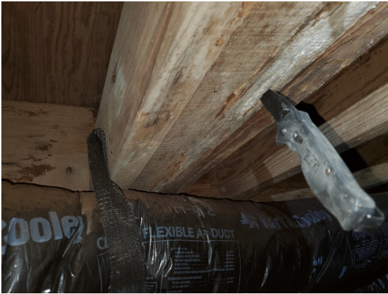
Picture 7 – Example of deteriorated beam
