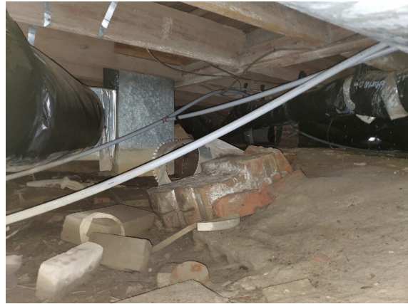
Picture 14 – Failed pier
