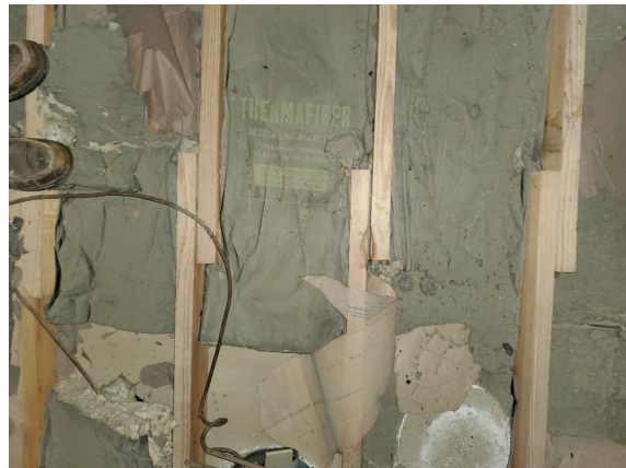
Picture 4 – Minorly twisted/rotated ceiling joists
