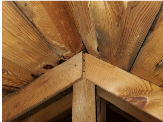
Picture 2 – Gaps between top chords
