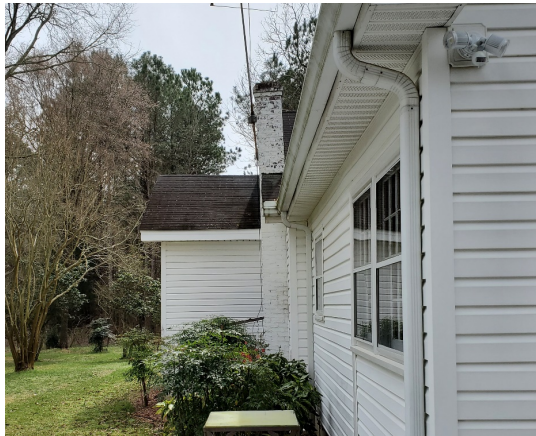
Picture 9 – Chimney visibly leaning
