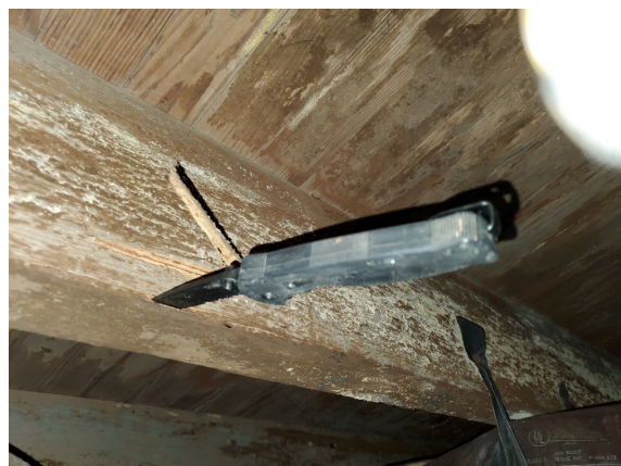
Picture 6 – Example of deteriorated joist
