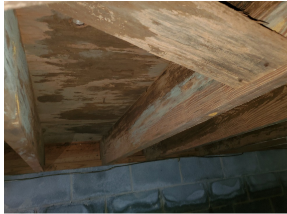
Picture 8 – Example of fungal activity
