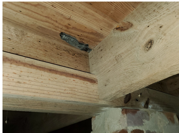
Picture 16 – Example of sagging ledger strip
