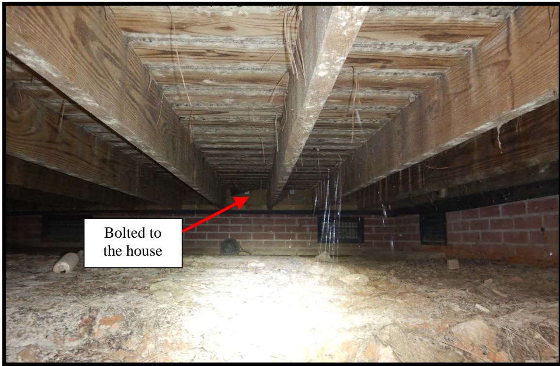
Photo #3 - This photo shows the band board was bolted to the house.
