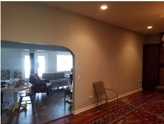
Picture 3 – Back dining room wall
